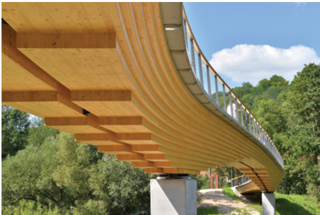
View of the underside showing the construction of the wooden superstructure (Fotograf Walther)
